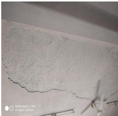
plaster shed off floor top
