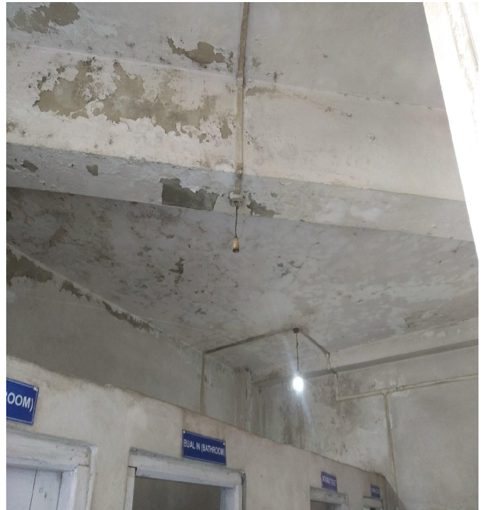
seepage on ceiling & all walls in toilet complex
