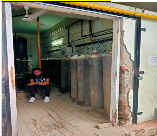
Damaged Plaster at Entrance of Manifold Room
