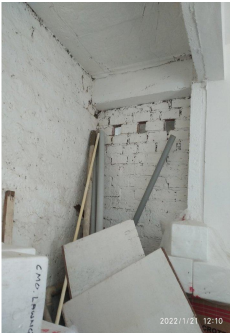
No plaster on right side wall portion OPD
