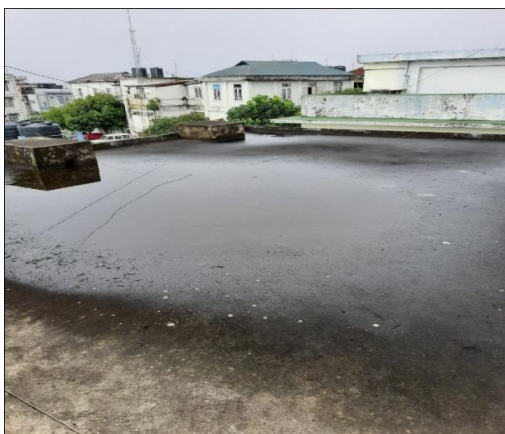
Block F Librarian room , Terrace waterlogged, need to be treatment area apex 5.2x5.2
