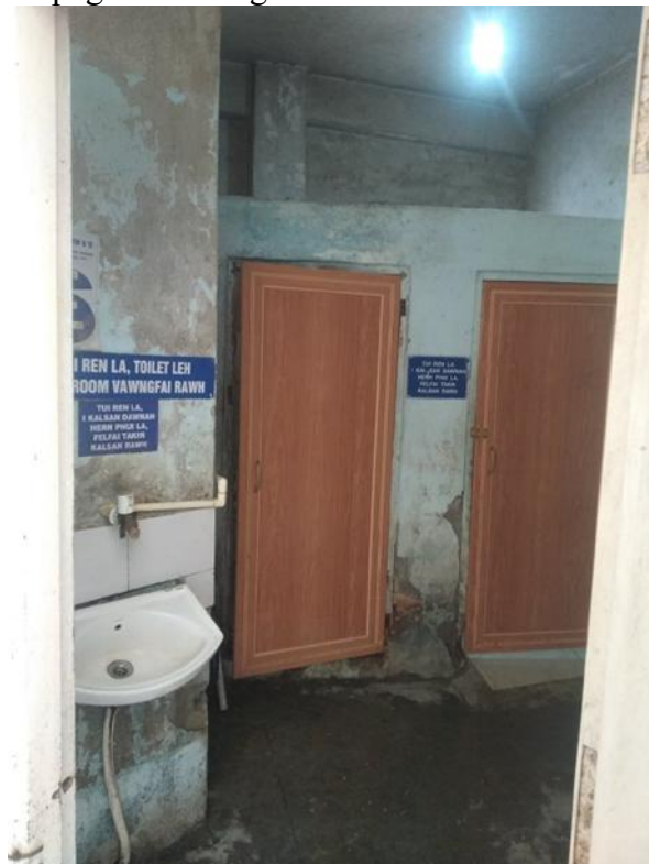
Brick work of toilets damaged in toilet complex orthopedic ward at second floor
