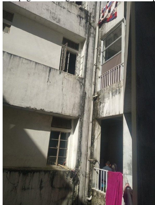
water leakage from drainage pipes near
