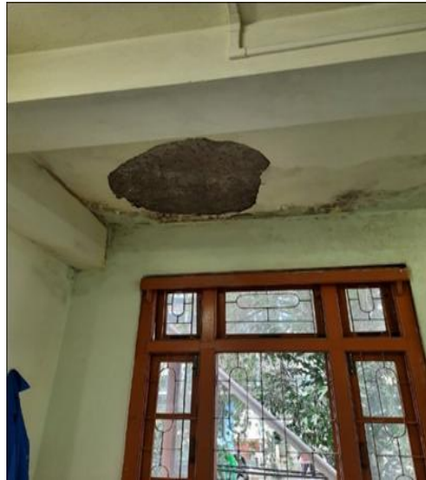
Block C-Third Floor Internal Ceiling Cracked, need Plaster Repair
