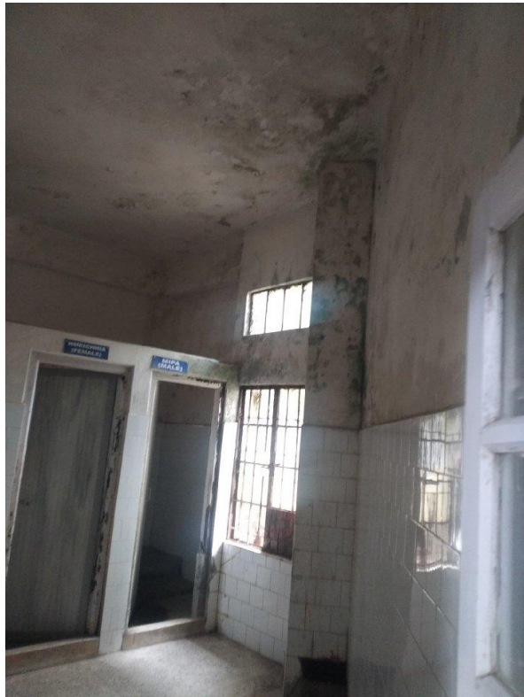
seepage on ceiling & walls in toilets.
