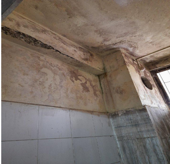
Block E Ceiling & wall seepage from shaft, and roof beam cracked, 2.4x1.2
